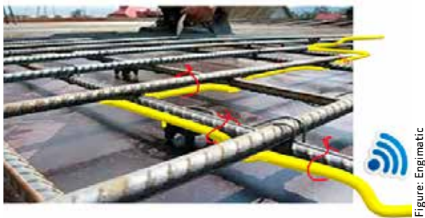
Fig. 5: The humidity sensors of the cable must have been fixed to the reinforcement before concrete placement
